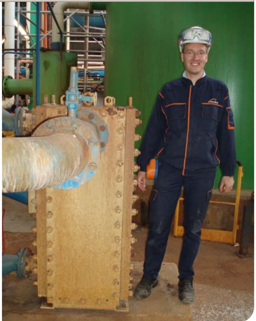
Emmanuel Corrado, production manager at Arkema's VCM plant, shows off the Alfa Laval Compabloc heat exchanger.
